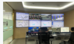
Energy Control Center
